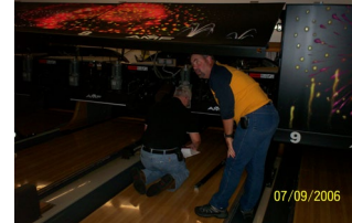
Don Wollek and John Schultz preparing to crawl under pin deck to measure lanes
